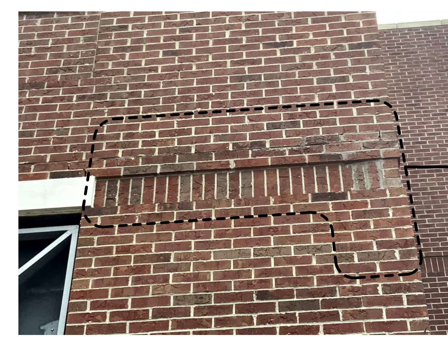
12 REPAIR / REPLACE DAMAGED UNITS. REMOVE AND REPOINT CRACKED MORTAR.
