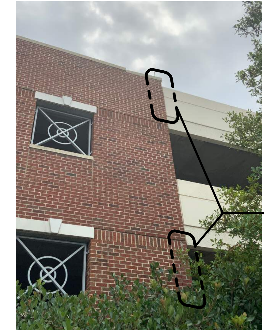
3 REPAIR / REPLACE DAMAGED UNITS. REMOVE AND REPOINT CRACKED MORTAR.
