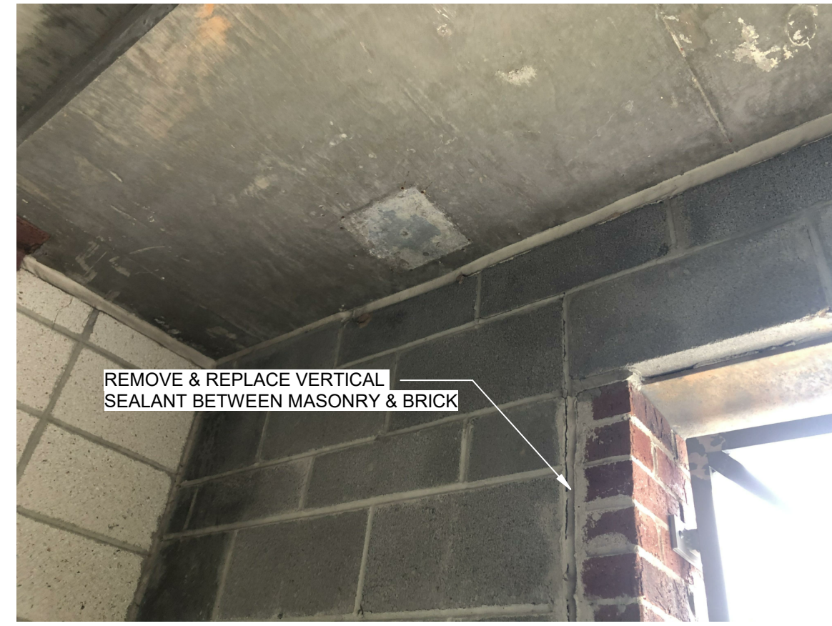
REMOVE AND REPLACE VERTICAL SEALANT BETWEEN MASONRY & BRICK 35.7 REPLACE VERTICAL SEALANT BETWEEN BRICK & MASONRY AT WALL OPENINGS
