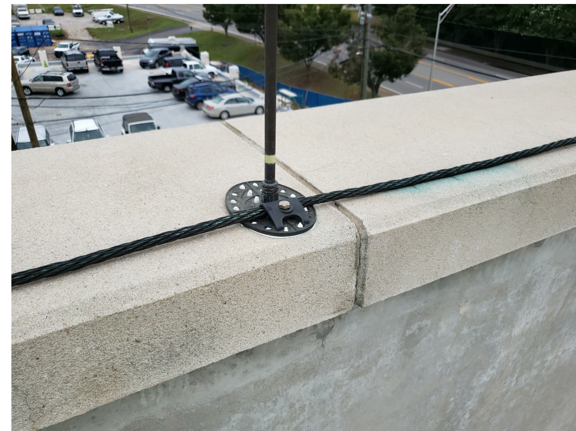
44.11 REATTACH LOOSE LIGHTNING PROTECTION AIR TERMINAL CONNECTIONS
