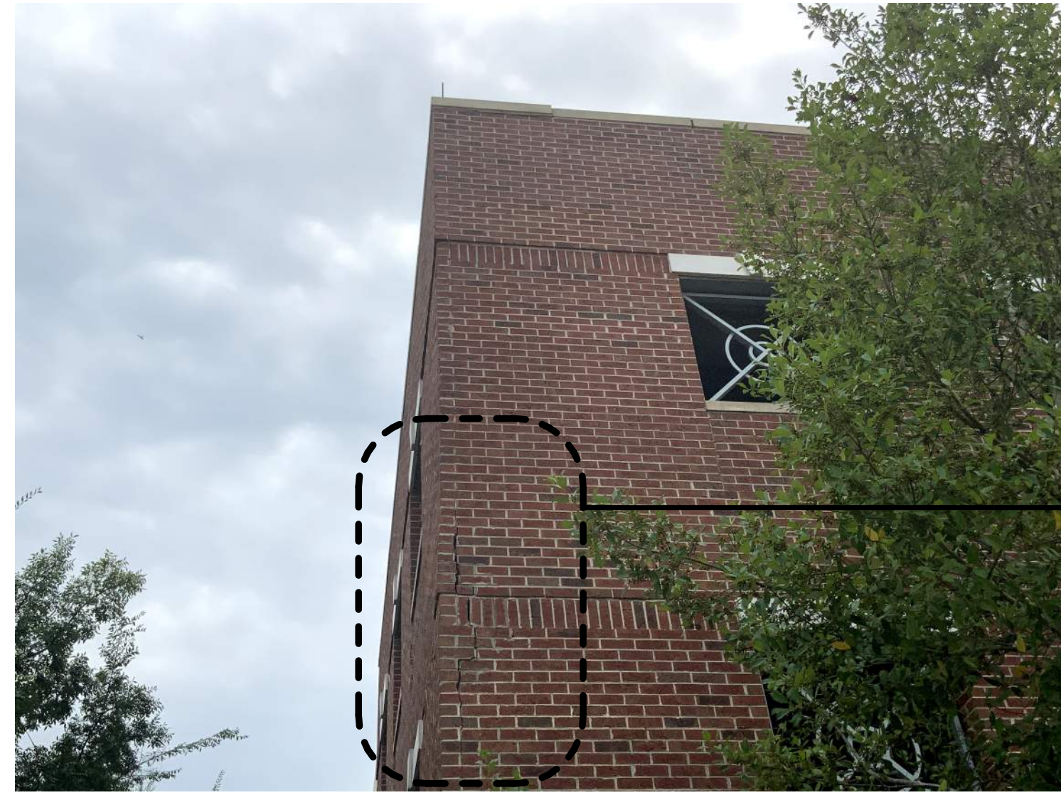
1 REPAIR / REPLACE DAMAGED UNITS. REMOVE AND REPOINT CRACKED MORTAR.
