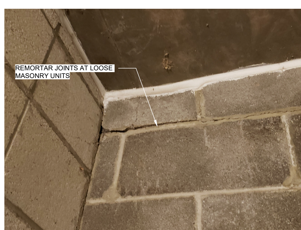
RE-MORTAR JOINTS AT LOOSE MASONRY UNITS
