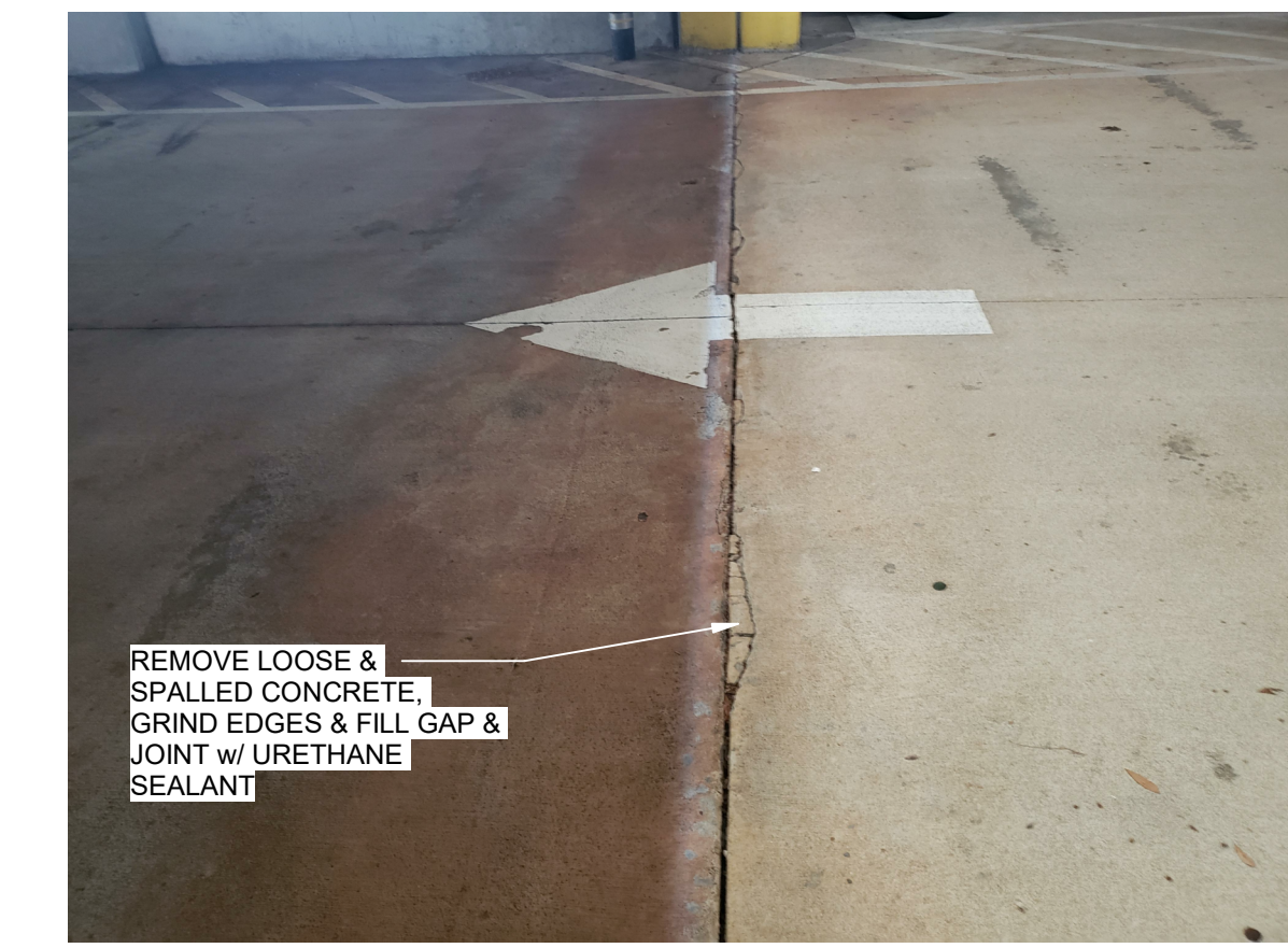
3.12 FLOOR REPAIR - SPALLED CONC. JOINT AT SLAB-ON-GRADE
