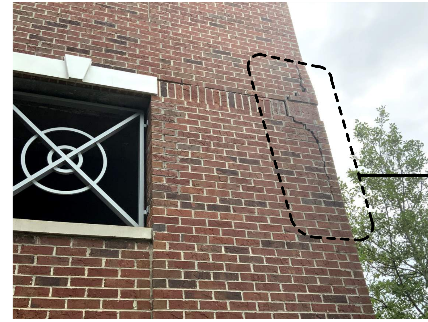
6 REPAIR / REPLACE DAMAGED UNITS. REMOVE AND REPOINT CRACKED MORTAR.
